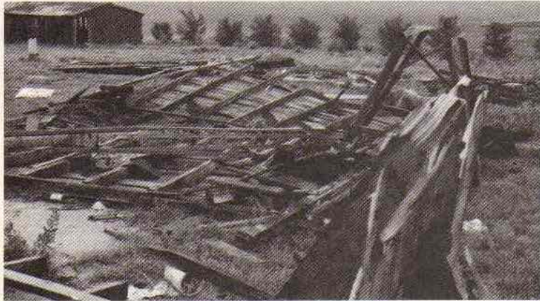
CONTACT reader Jennifer Vratil took this photo of a building damaged by a tornado.
